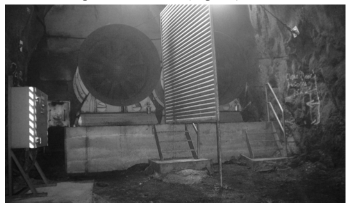
Figure 11. Baffle between parallel fans
