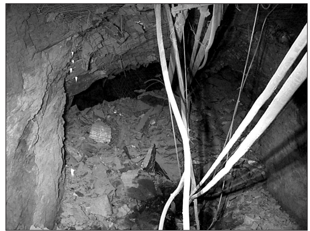
FIG. 5 Photograph looking west, showing the eventual failure of the back of the 7350 x/c on 15B Sublevel at the point adjacent to stope H742, conditions compounded with I73 orepass breaching the cross-cut
