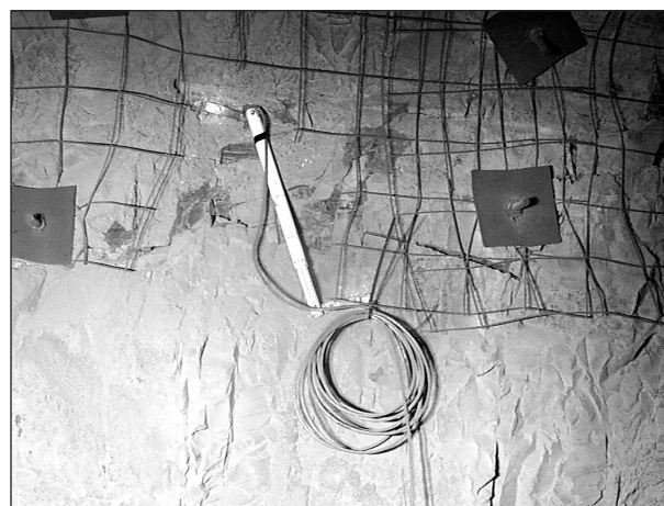
FIG. 3 Photograph showing one of several crack extensometers monitoring the intact rockmass failure in the sidewall of a north-south striking drive on 6 Level. The drive is adjacent to a series of unfilled stopes (the ground was slowly moving towards the voids and subsequently 'tearing' the rockmass apart in tension)
