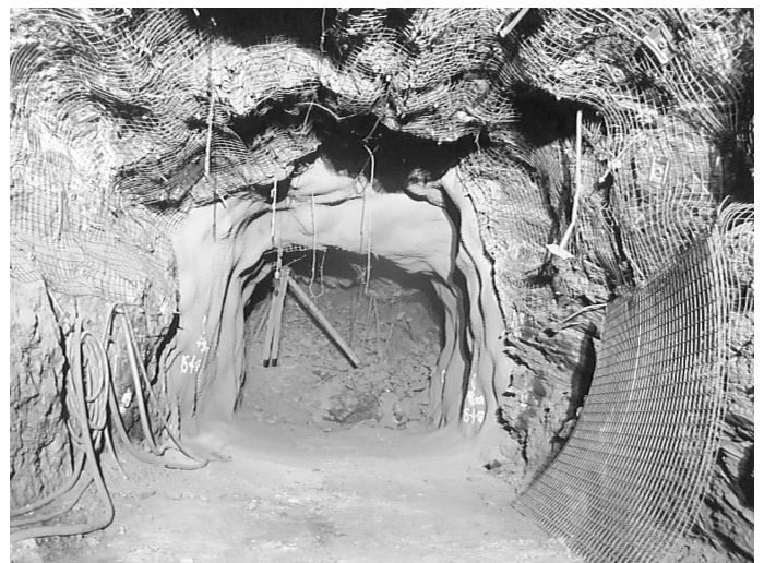
Figure 6. Looking south along P3849 SEDR (20B) at the first stage of the initial rehabilitation process, with the spraying of shotcrete (150 mm) and prior to the installation of the reinforcing cable bolts.
