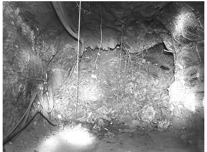
Figure 5. Looking south at the fall of ground at the point of arresting, at the intersection of P3849 SEDR and Q369 CO, 20B Sublevel.
