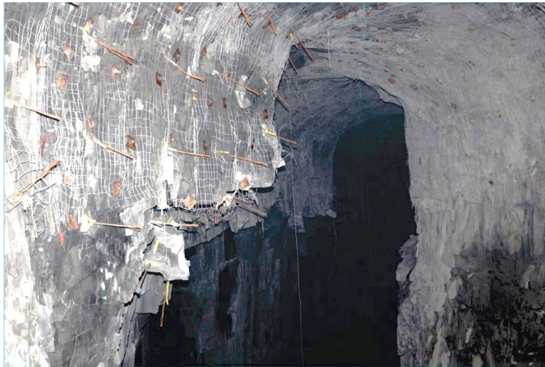
Figure 10. This picture shows the damage produced by the tight pattern (2.3 m, 7.5 ft x 2.0 m, 6.6 ft).
