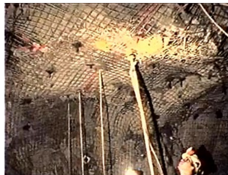
Frame 2 – Wedge assembly positioning with a blasting pole that acts like a giant screwdriver. Note that there are 3 wedge installations already set.
