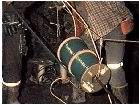
Frame 2 – Loading 2 stands of Primaflex into shear boreholes using the wedge/pulley/rope method.
