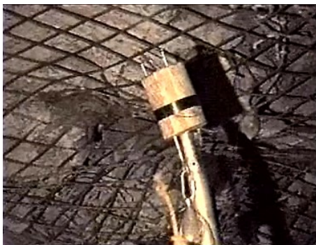
Frame 1 – Wedge assembly ready to be inserted into shear borehole. A borehole camera would be used to ensure that the wedge had expanded to the shear borehole wall.
